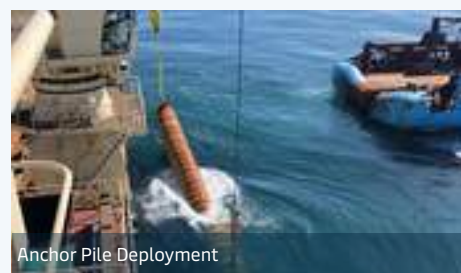
Anchor Pile being over boarded by the two cranes aboard Maersk Inventor
